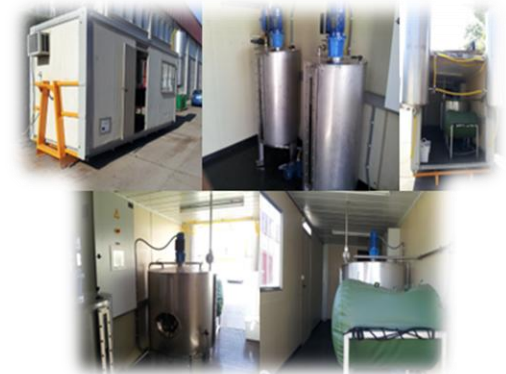
Figure 6.- Biomethanization pilot plant
